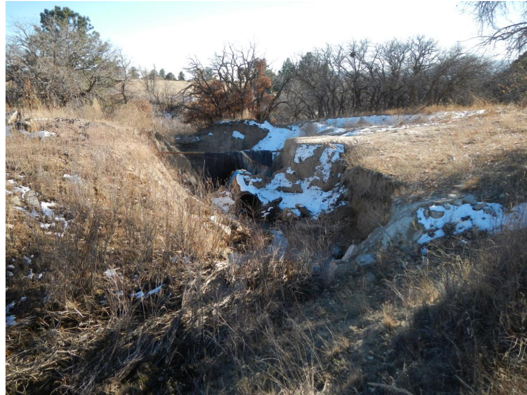
Figure 36. MT-1: Stabilize Headcutting on Middle Tributary South of Middle Creek Parkway
