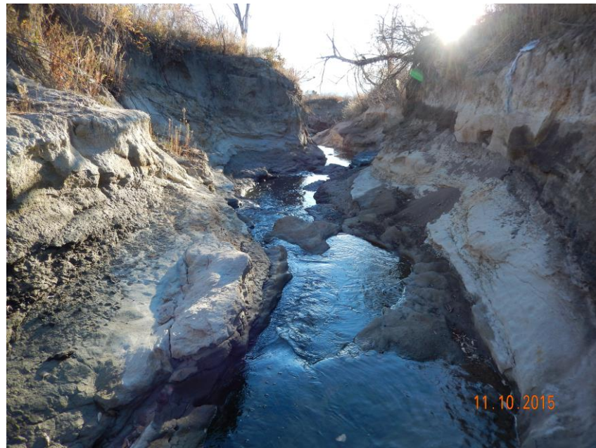
Figure 50. PC-7: Pine Creek Small Drop Structures East of I-25 and Downstream of Academy Boulevard
