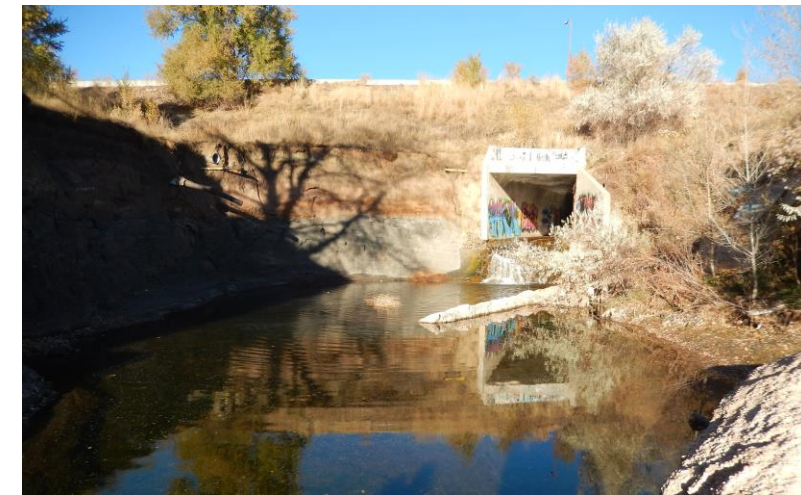
Figure 13. NDC-2: North Douglas I-25 Downstream Failed Wingwall and Erosion
