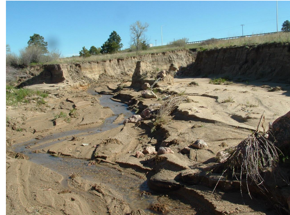
Figure 15. MB-3: Monument Branch Tributary Erosion between Northbound and Southbound I-25
