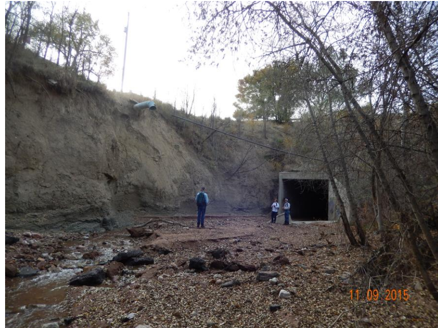
Figure 14. SDC-3: South Douglas I-25 Downstream Failed Wingwall and Erosion
