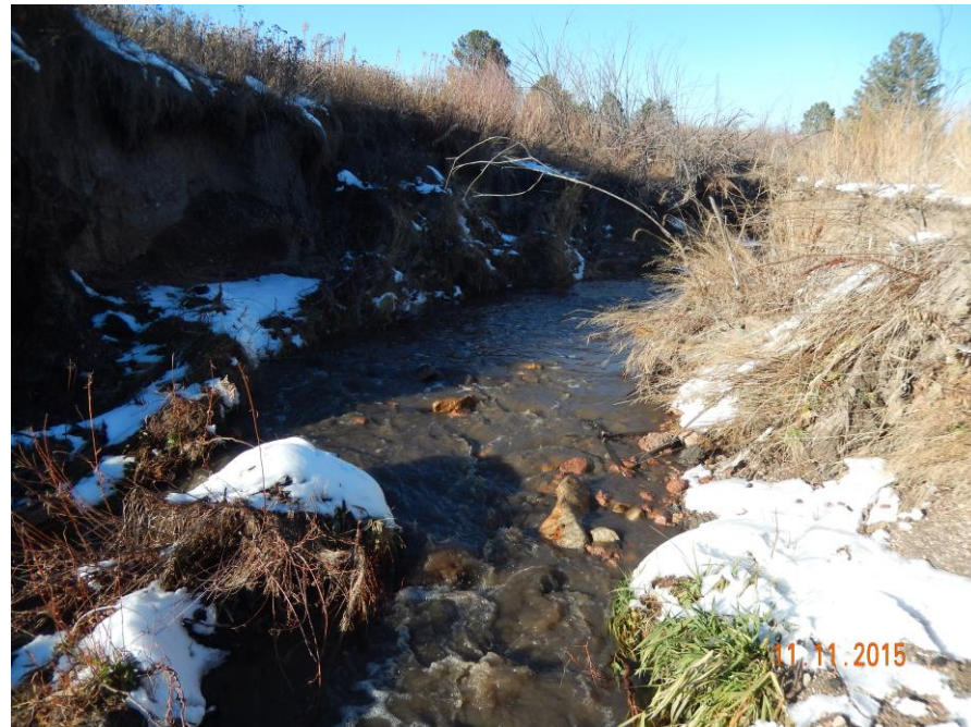
Figure 24. JC-1: Jackson Creek Small Drop Structures East of the Monument Creek Confluence
