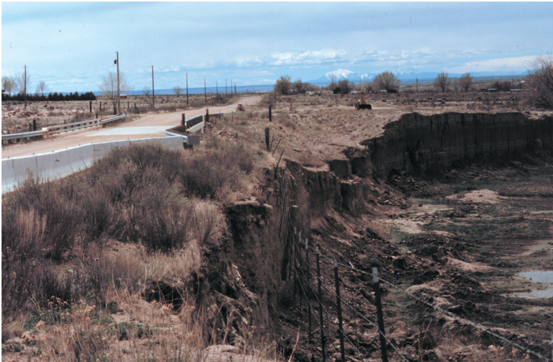
Figure 15. View looking south at the Overton Road bridge and edge of high terrace on April 26, 1999. Following the flood of April 28 through May 5, Overton Road at this location was reduced to one lane due to bank erosion after which the edge of the terrace extended a few feet into the southbound lane from the near foreground to the bridge.
