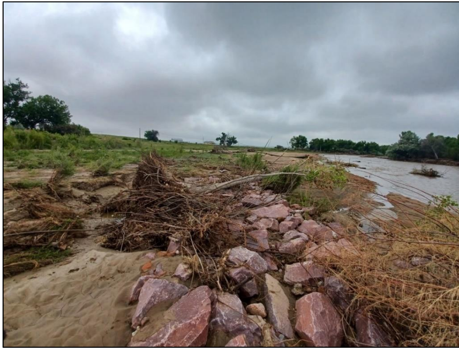
Figure 11. Riprap bank protection buried by sediment.
