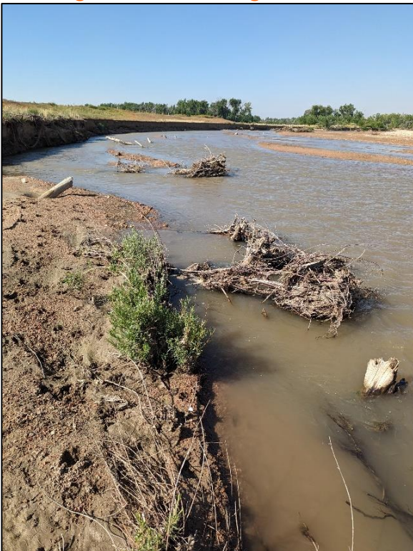
Figure 23. Damaged Toe Wood
