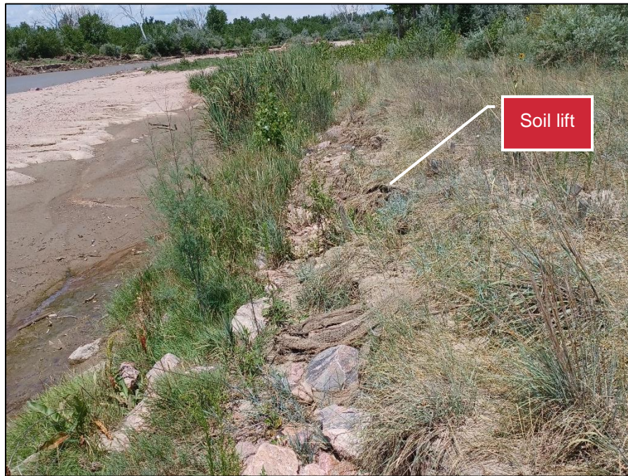
Figure 28. Riprap bend protection and soil lifts
