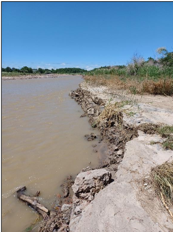
Figure 35. Bank erosion, typical to the site.
