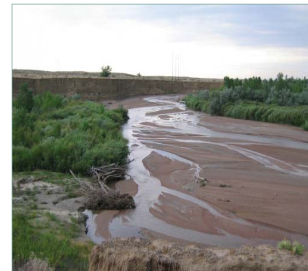
Fountain Creek at Williams Creek confluence, downstream view on Frost property of aggrading channel reach with large cut bank. Photo courtesy of URS Corporation
